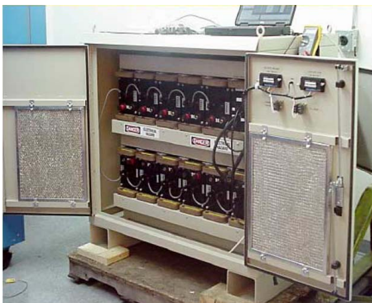
Figure 3: A 100 kW Li-ion energy storage system
